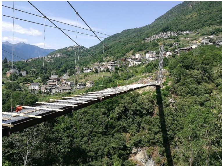
Fig. 13. Deck installation and preliminary works for the installation of the stabilization cables
