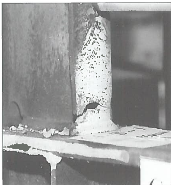
Fig. 7 Typical failure mode, with weld cracking.
