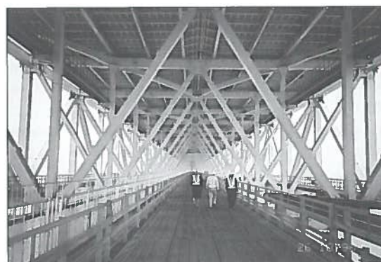
Akashi Bridge: hosts and guests on route from the south anchorage to the south tower, along the maintenance lane on the wide steel grid platform at the lower level of the deck, used also by maintenance vehicles. (Photo: Juhani Virola)
