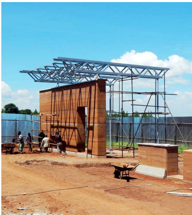
Fig. 16 – Vista del mock up della muratura in pisé. © Emergency NGO Technical Department
